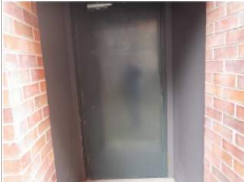
Encl 16 - Metal Swing Doors
